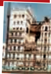
» The Brighton Grand Hotel suffered major damage when an IRA bomb attempted to assassinate Margaret Thatcher.
